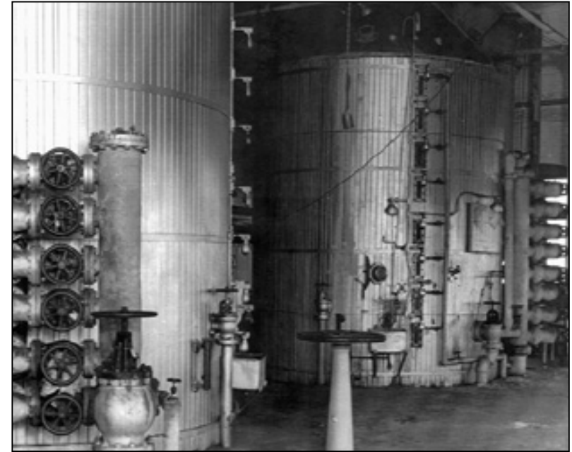
Vacuum pans located on the fourth floor. Purified sugar was boiled in vacuum pans to create sugar crystals.
